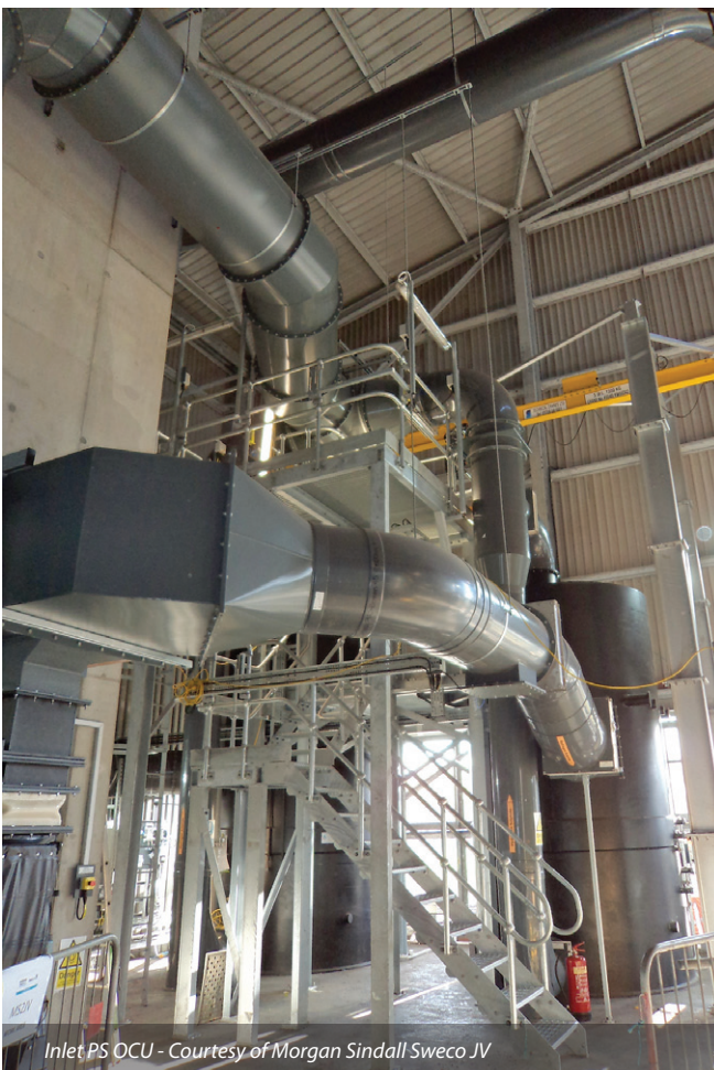
Treatment at source plant - Courtesy of Morgan Sindall Sweco JV
